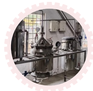
Small Scale essential oil Distillation Plant
